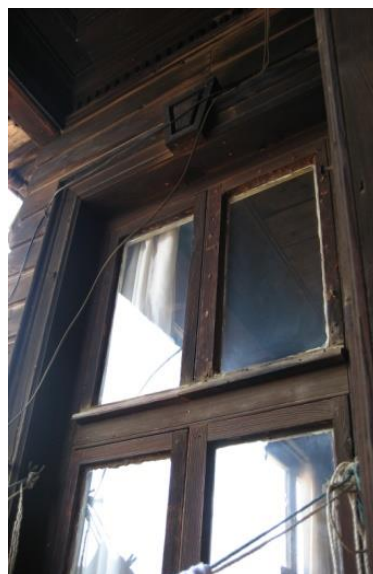
Figure 11. Cepneli Mehmet Bey house– Window detail (P. A.)
